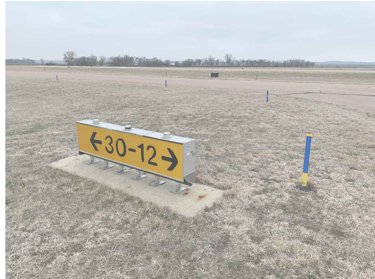
EXISTING AIRFIELD UNLIGHTED SIGN W/ CONCRETE SIGN PAD
